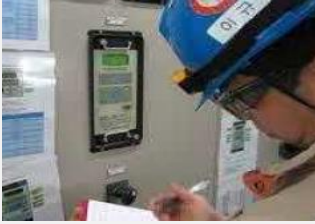
Maintenance inspections by humans on foot/with the naked eye/record the results manually
